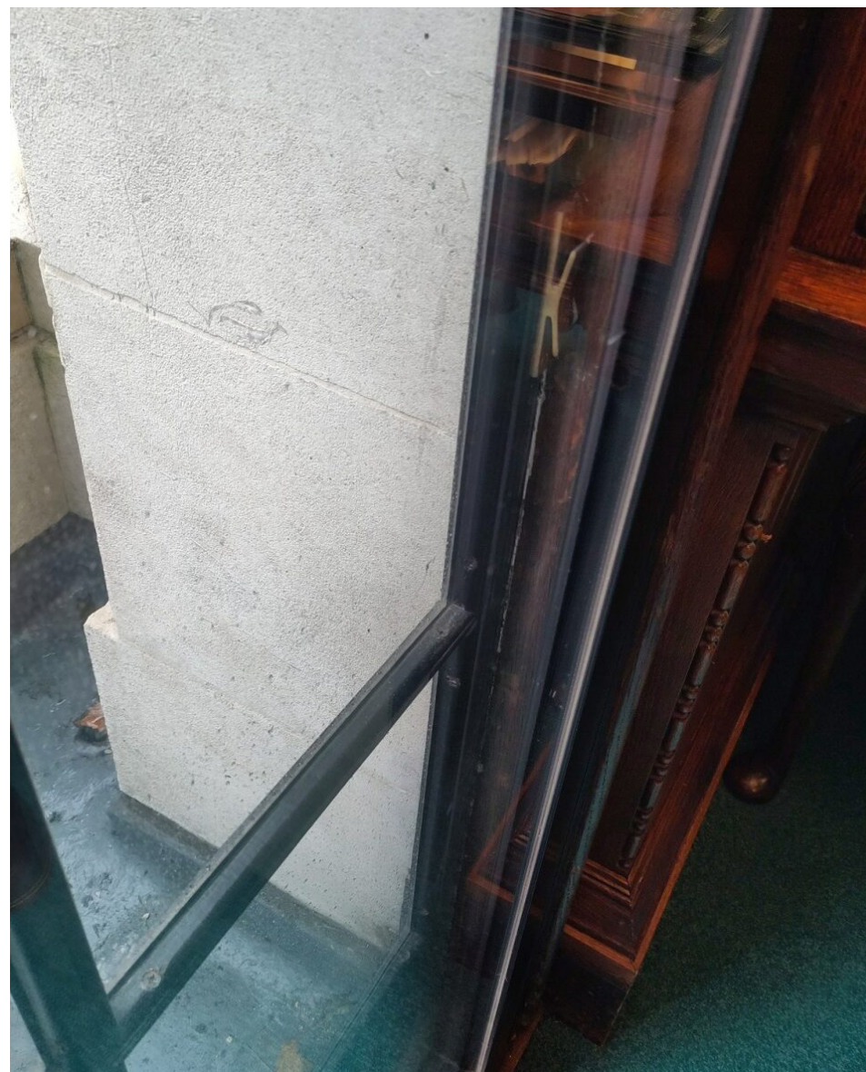
Image 6. Secondary glazing carefully chosen to have minimal impact on the listed fabric and significance.
