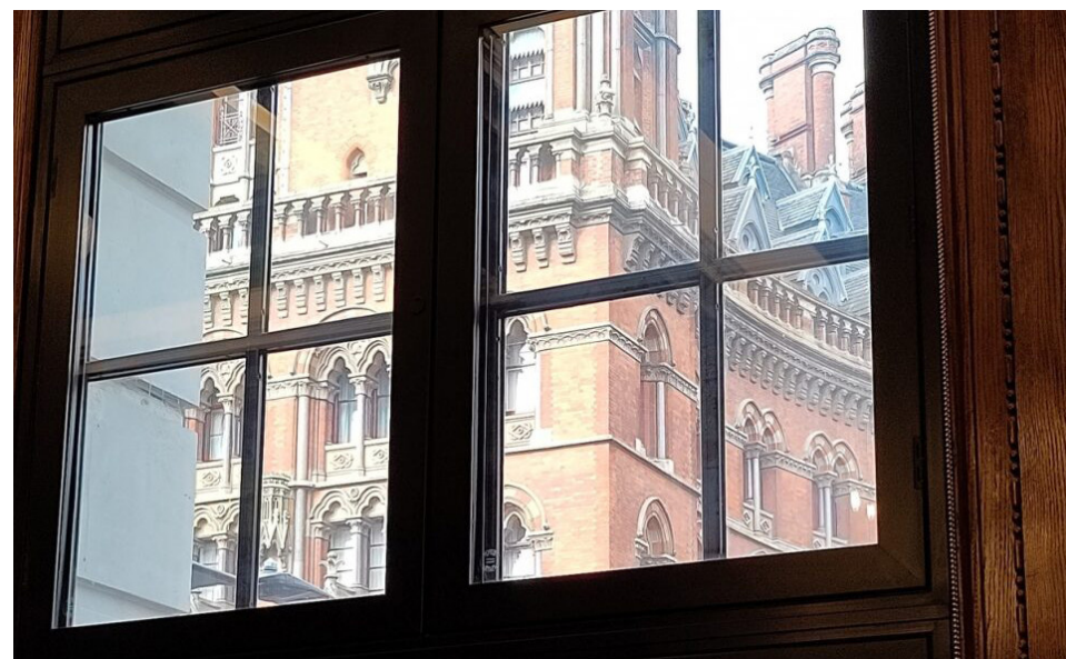
Image 5. Discrete secondary glazing installed in a listed building.
