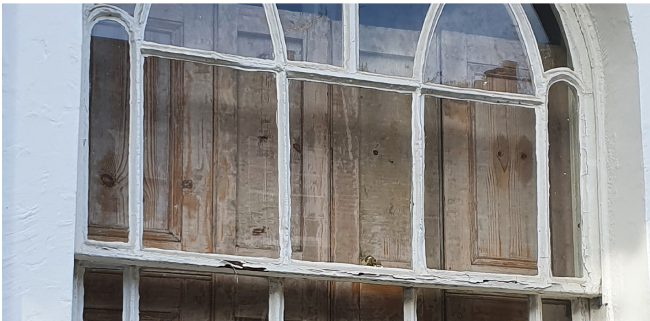
Image 4. Defects to paintwork and putty are common and can be addressed with routine repairs.
