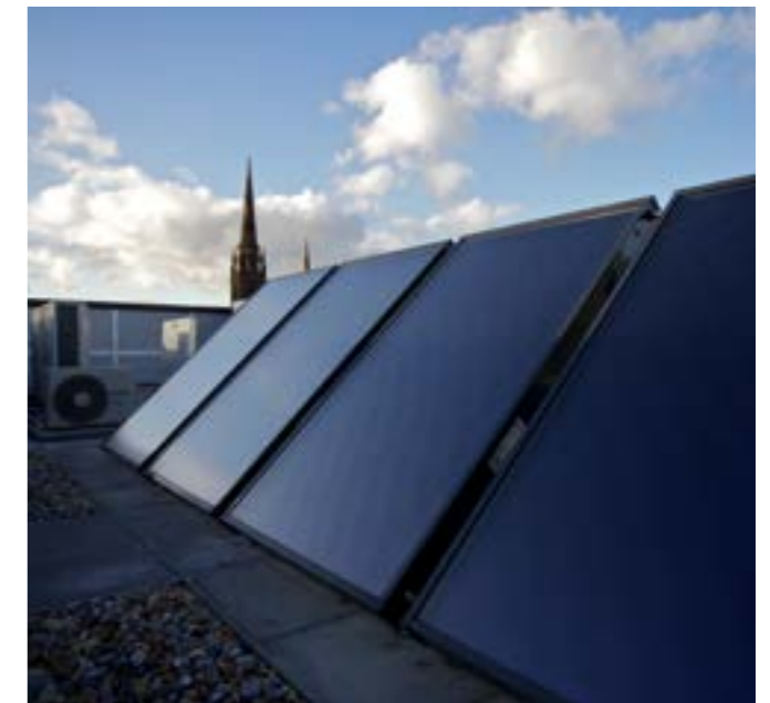
Image 2. Photovoltaic panels installed on a flat roof
