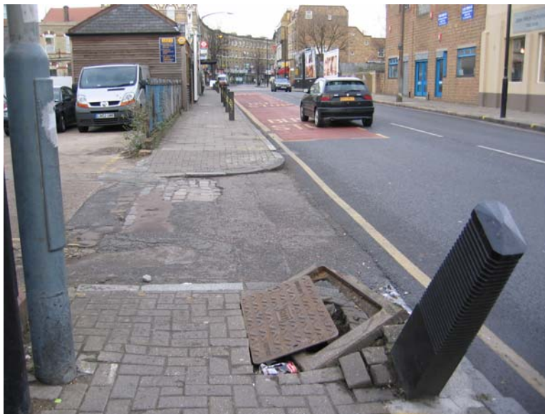
An example of a damaged piece of street furniture
